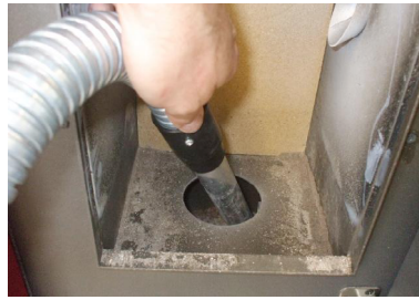
Fig. 38 - Burning pot box cleaning
