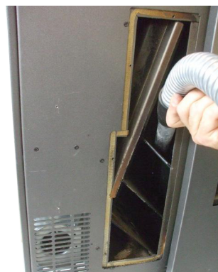
Fig. 44 - Fume chamber cleaning
