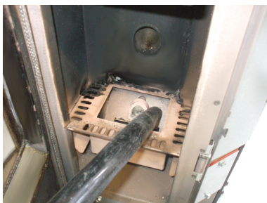
Fig. 36 - Burning pot box cleaning
