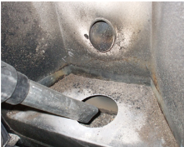
Fig. 33 - Burning pot box cleaning
