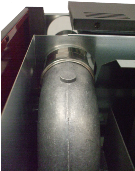
Fig. 33 - Rear pipes position
